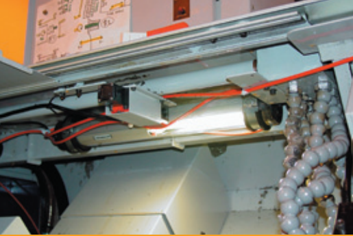
Red Firetrace Detection Tubing runs unobtrusively through the working area
